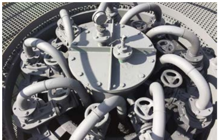
Image: PVEG50M manual polyamide body pinch valves in a hydrocyclone at Kara Mine, TMM, Tasmania, Australia.
